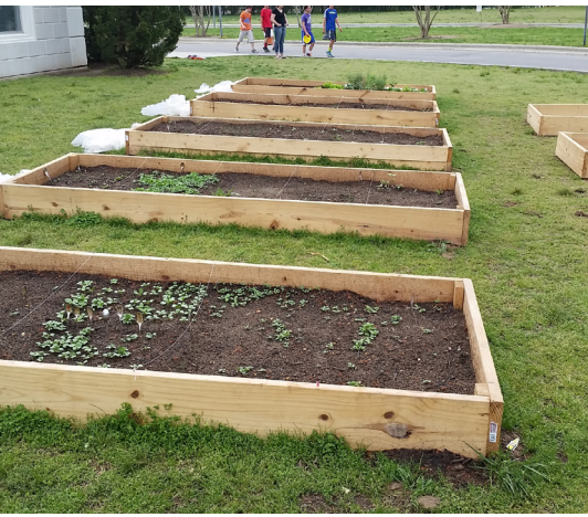
FIGURE 5-3 Using lumber already cut to length to make a raised bed. This requires few cuts and students of all ages can help build the beds.
